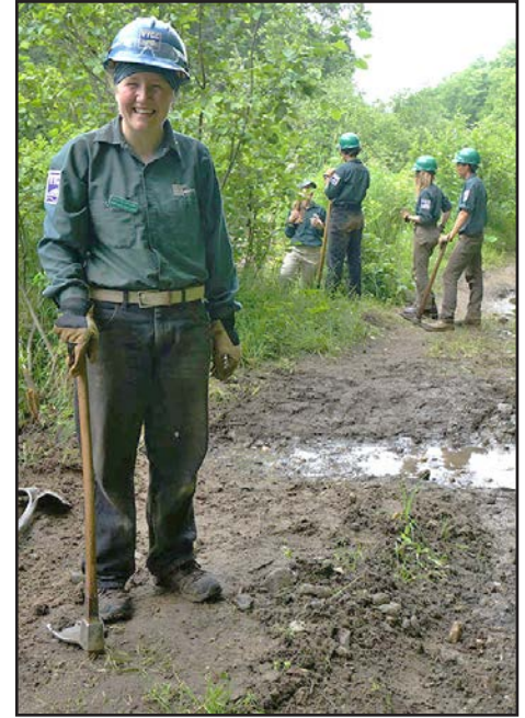
Caroline leads a Crew digging runoff channels along a low lying section of road along the East Elmore Branch of the Lamoille River
