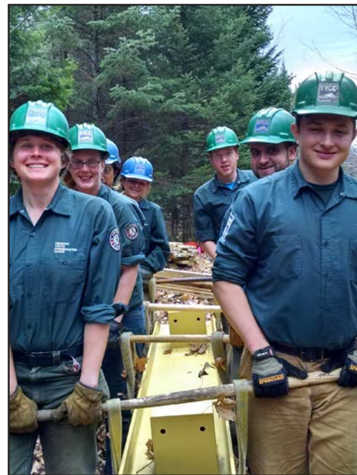
Seth (front right), Tinian (back left), and the crew of Cons 4 carry a steel I-beam to a bridge construction site in Jay
